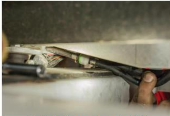
Fig 19c (Valve seen from the side)
