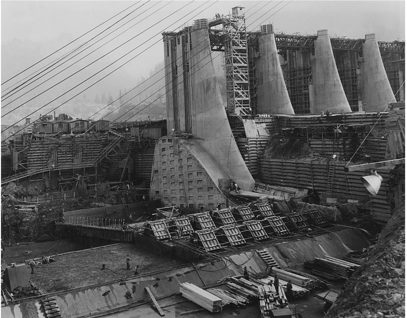
Public Works Administration Project, U.S. Army Corps of Engineers, Bonneville Power and Navigation Dam in Oregon, Columbia River, 40 miles East of Portland, "Downstream side of Blocks 7 and 8 of North Half of Spillway Dam and Piers 9 to 12. Inclusive of South Half of Dam," October 24, 1936 ( National Archives, Franklin D. Roosevelt Library )
