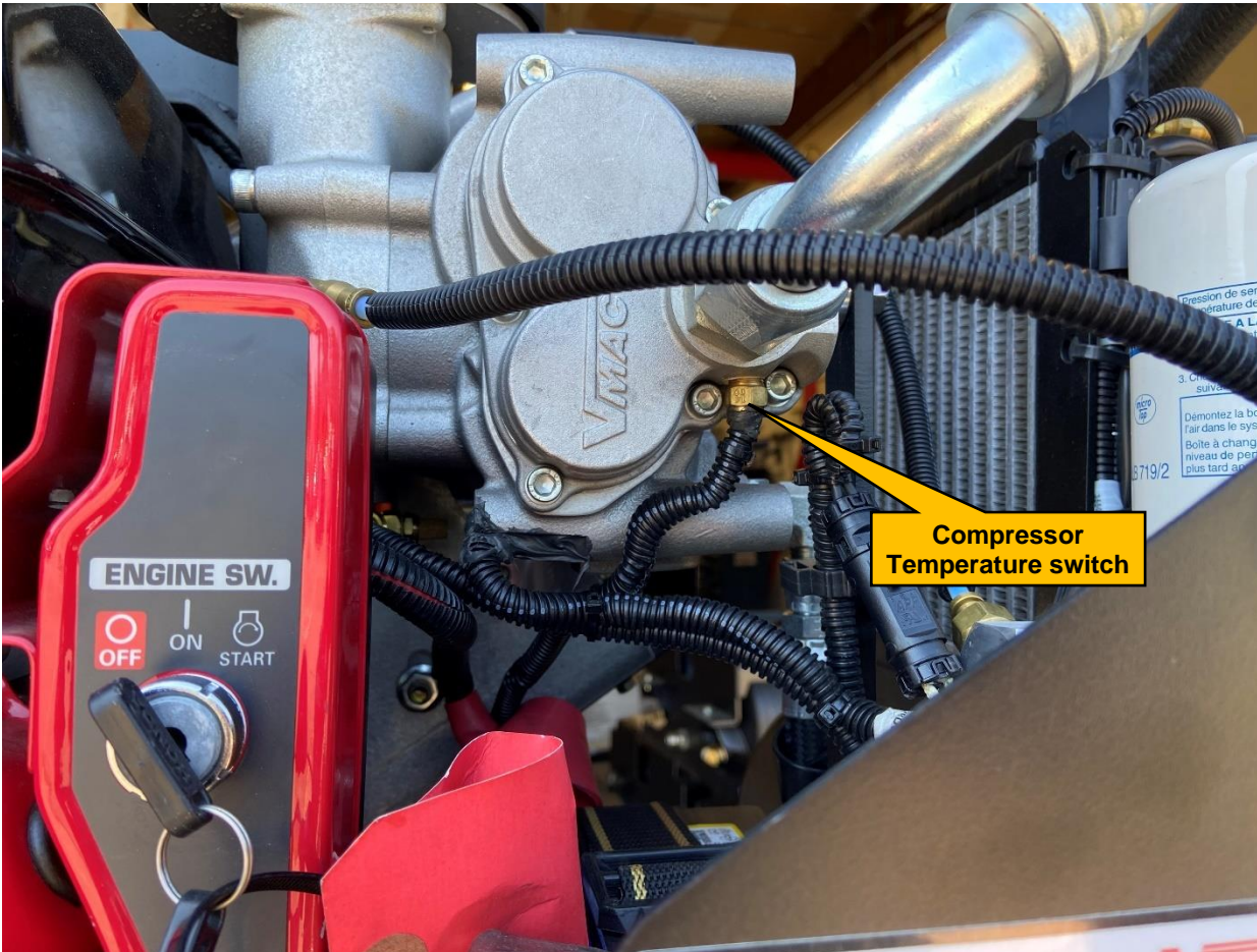
Compressor temperature switch
